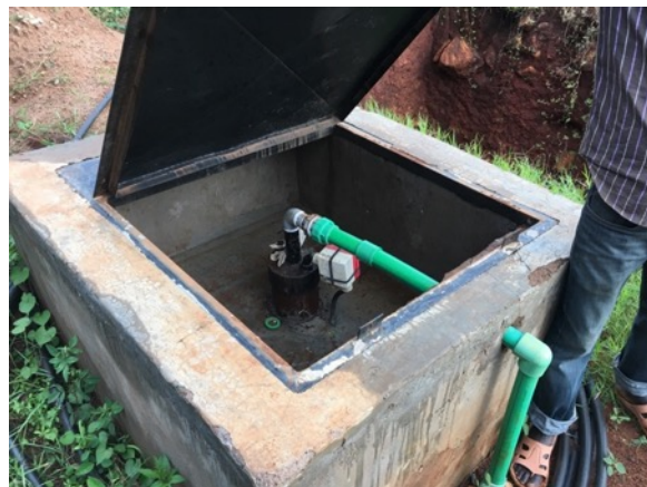
Figure 5.4: Private Electric Pump Installed by WECCO
