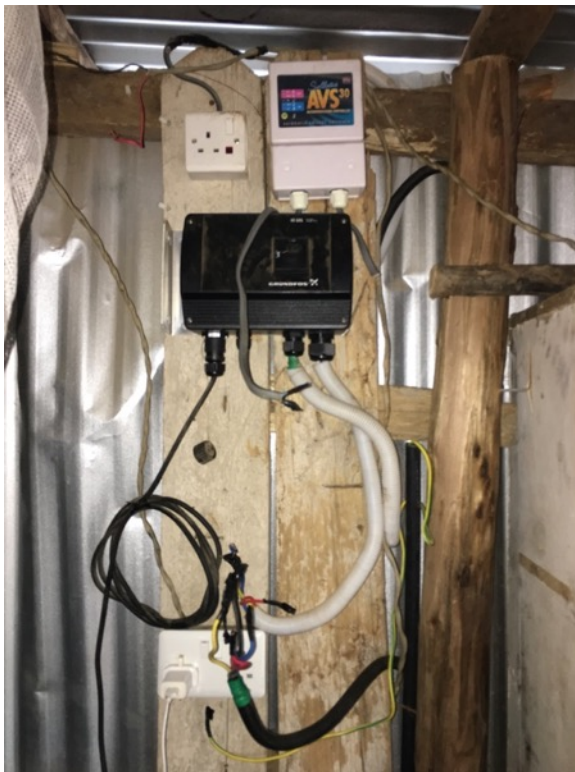
Figure 5.3: Electric Pump & Well
